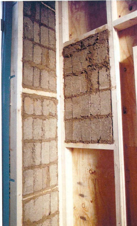
For earthquake-resistant houses in hot regions: a wood-frame wall filled with clay bricks
